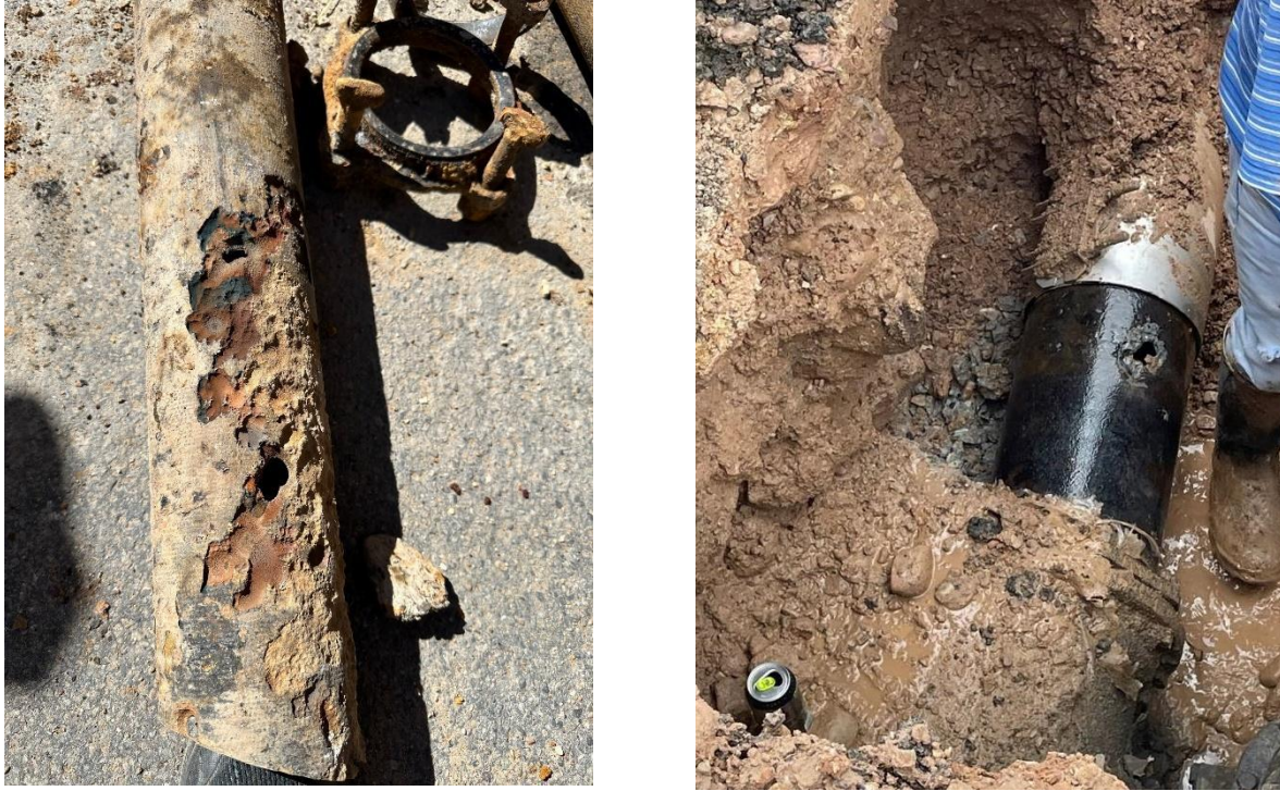
Figure 5, Severely corroded lateral water line (left), Main Street main water line repair (right). Source: PCMC, as of August 2023.
