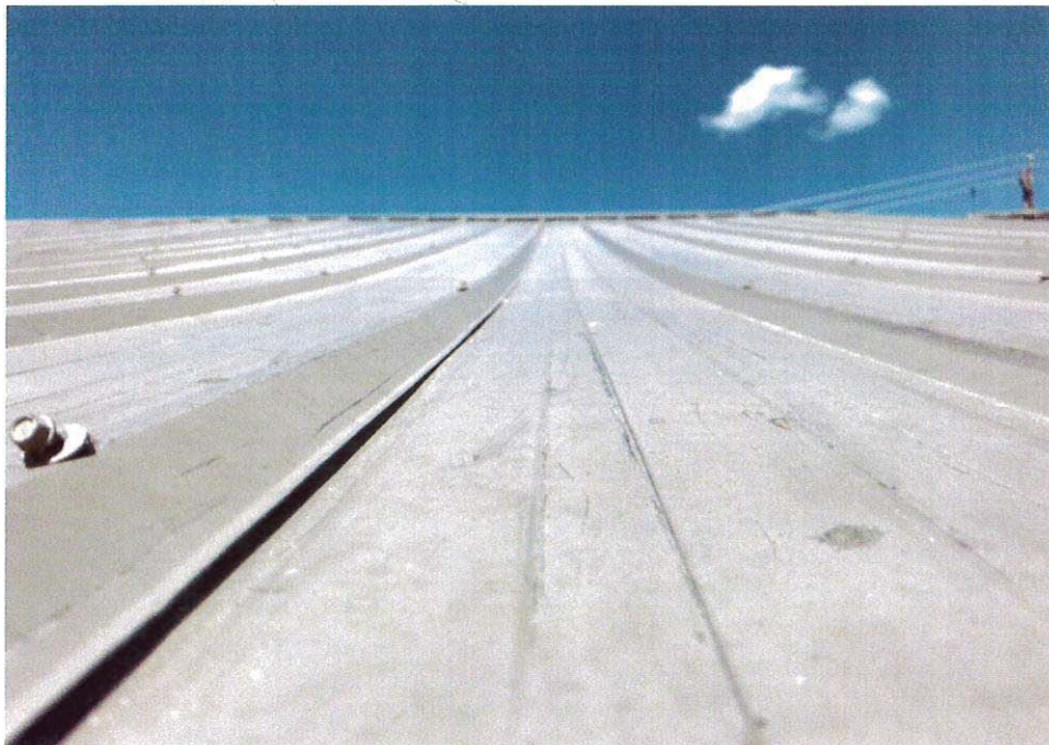
Photo 8: Ridge Sag and Joist Bow
