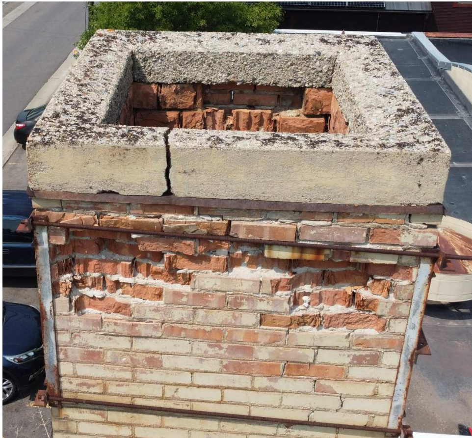
Figure 1: Large Crack in Cap Flashing and Damagved Bricks
