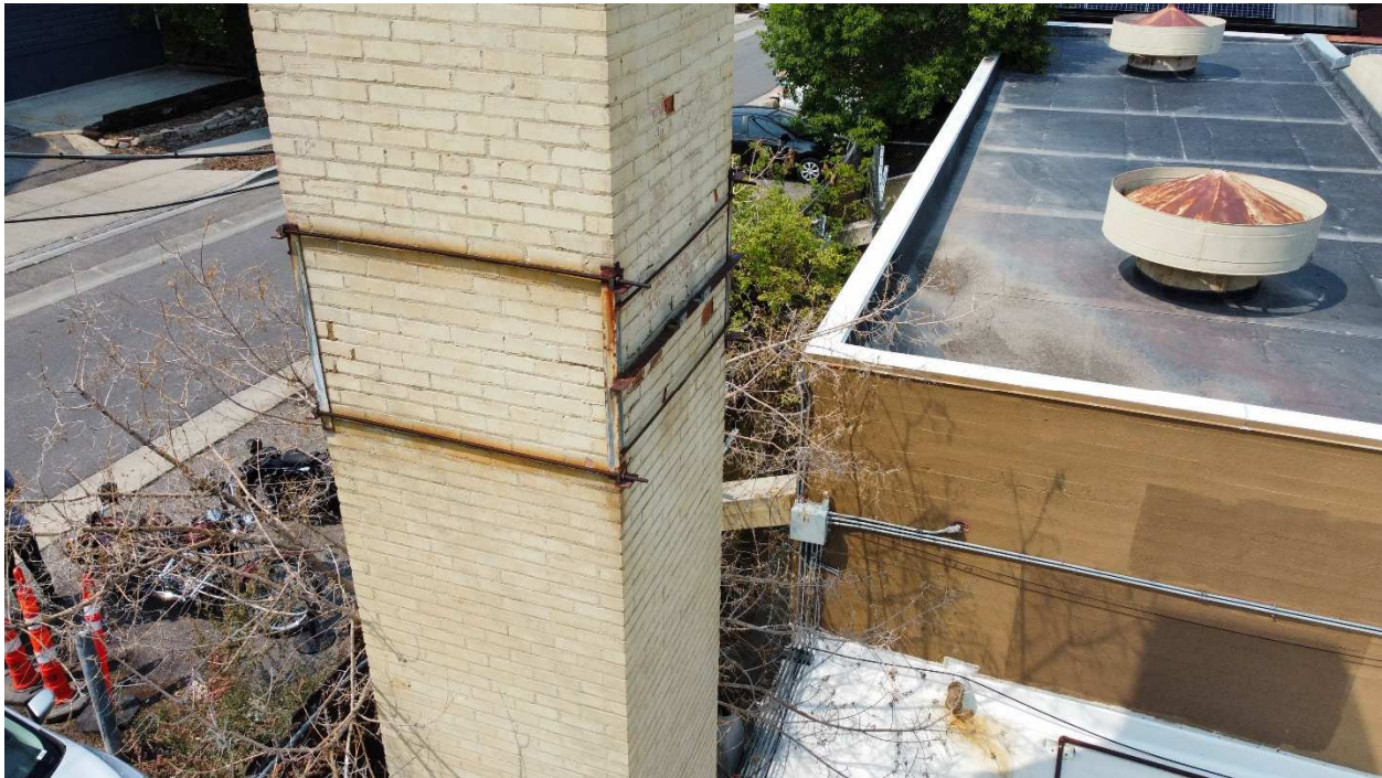
Figure 7: Mid-Section Reinforcing is not Enough for Seismic Loads
