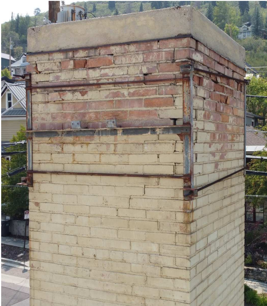
Figure 5: Damaged Bricks and Wall Cracking
