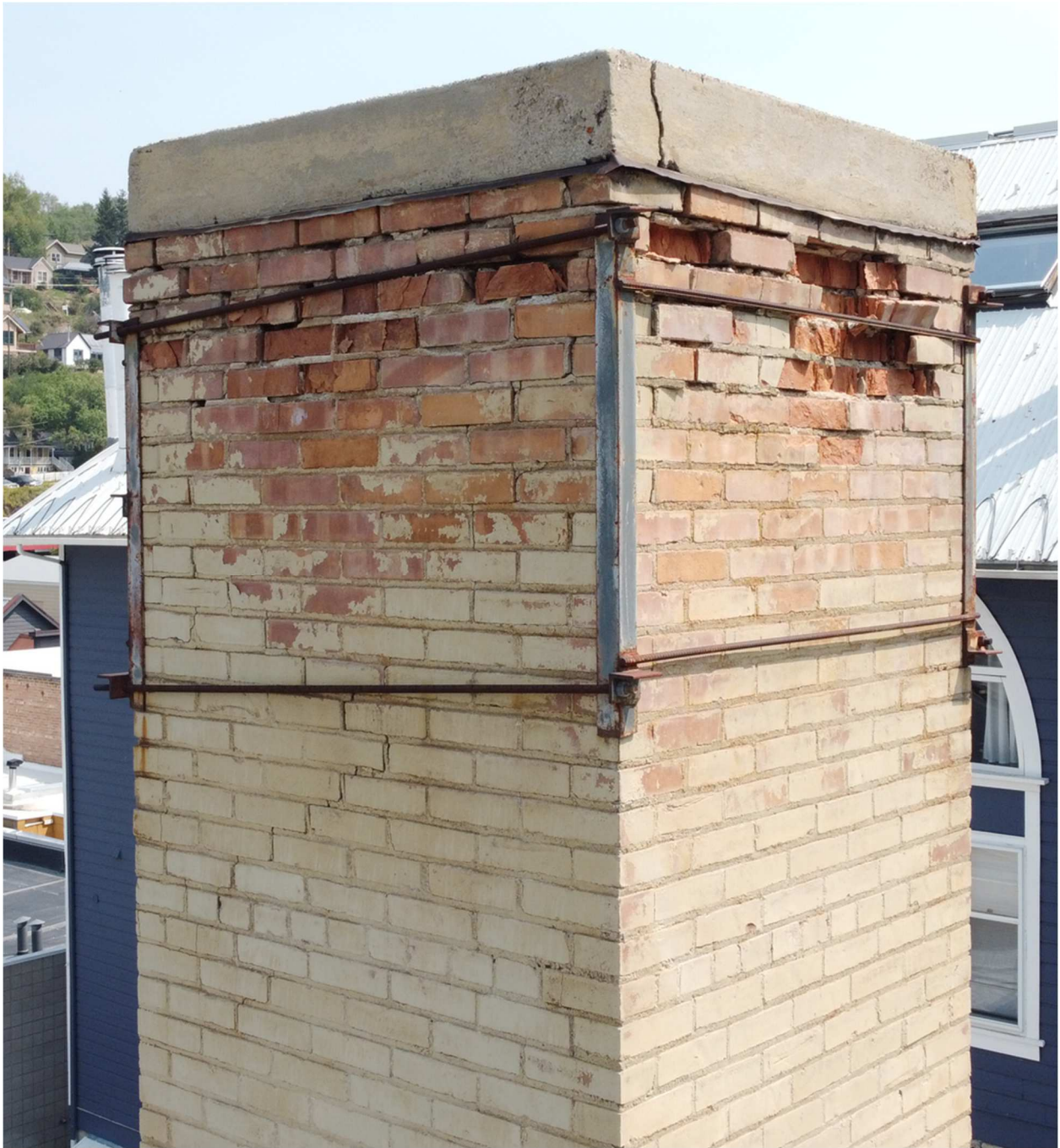
Figure 4: Large Crack in Cap Flashing and Damaged Bricks
