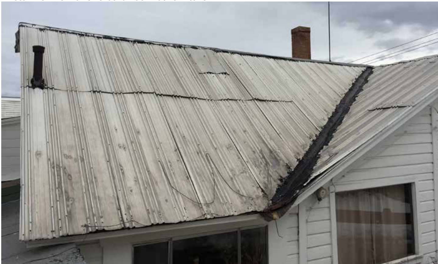
Photo #18: View of Overbuilt Roof Above Kitchen
