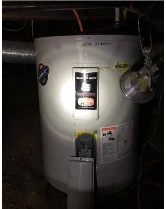
Photo #43: Water Heater In Crawl Space
