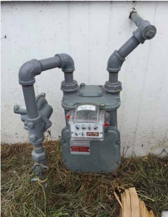
Photo #44: Gas Meter At Front Of House
