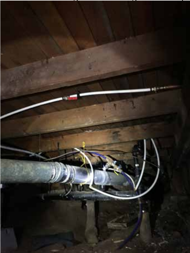
Photo #46: Ducting and Plumbing in Crawl Space
