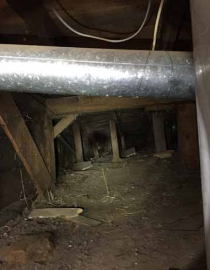
Photo #37: Crawl Space W/ Lack of Foundation
