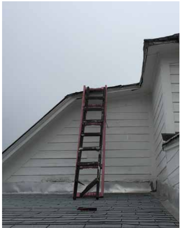
Photo #32: Left Side Overbuild
