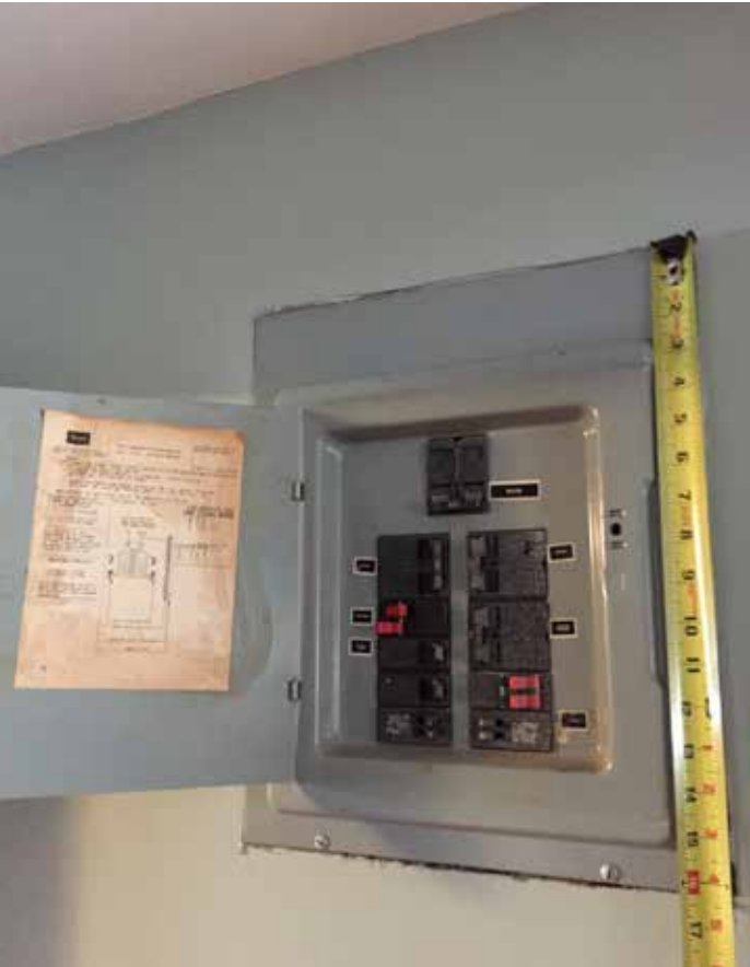
Photo #47: Electrical Panel In Kitchen
