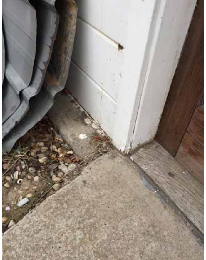
Photo #36: Exposed Foundation At Addition
