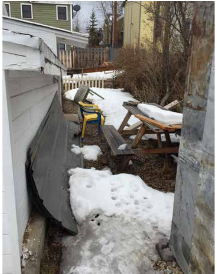
Photo #6: Rear Yard Grading
