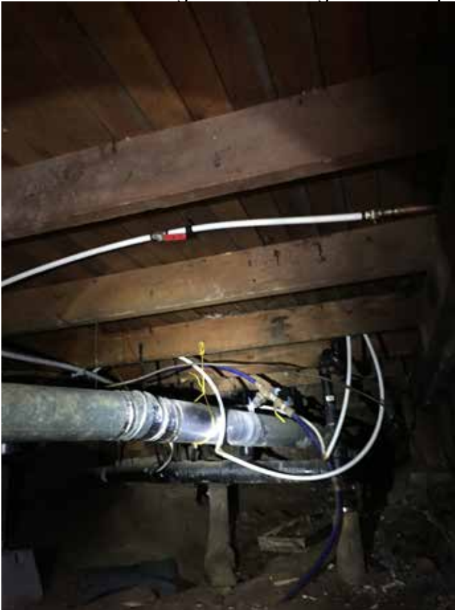
Photo #46: Ducting and Plumbing in Crawl Space
