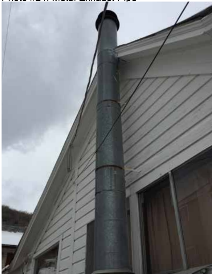
Photo #24: Metal Exhaust Pipe
