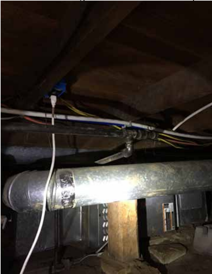
Photo #42: Heating Unit On Side In Crawl Space
