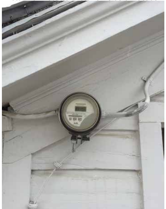
Photo #45: Electrical Meter On Side of Facade
