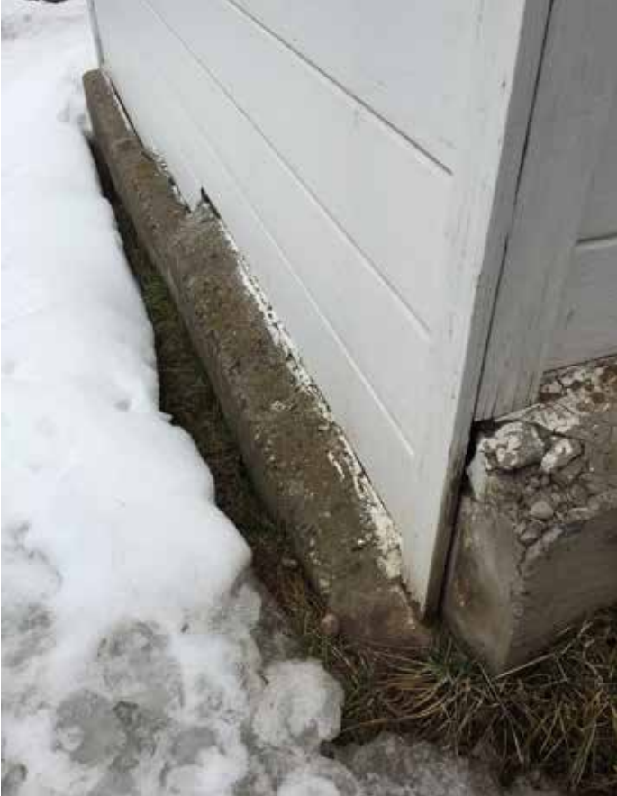
Photo #35: Exposed Foundation At Addition
