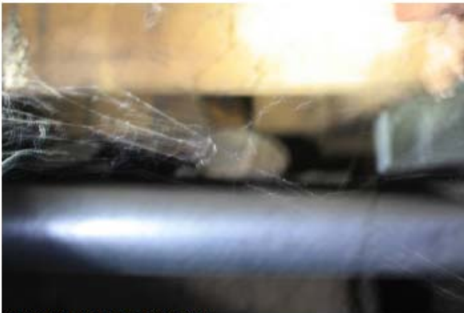
Duct work-exposed no insulation
