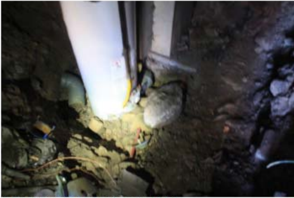
Damage to existing foundation-rubble fallen
