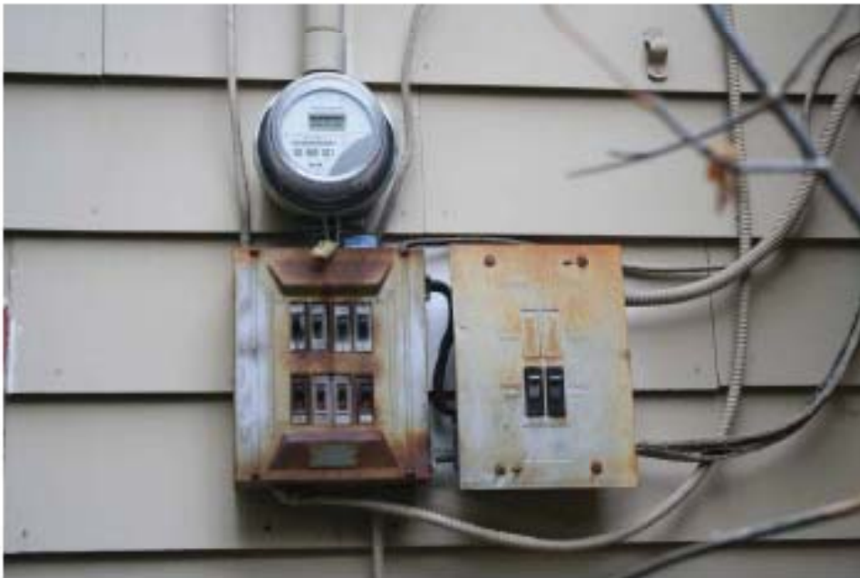
2. Closeup electrical service
