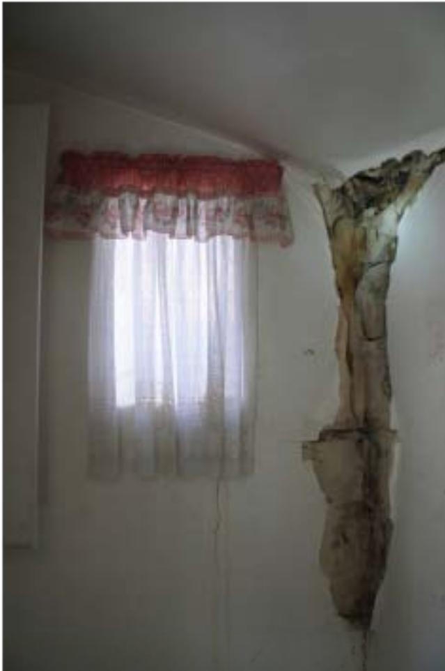
Visible mold-probably hidden mold
