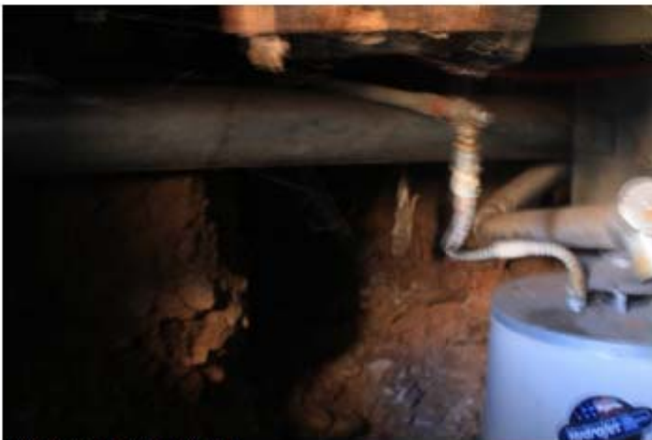
Hot water heater-venting?
