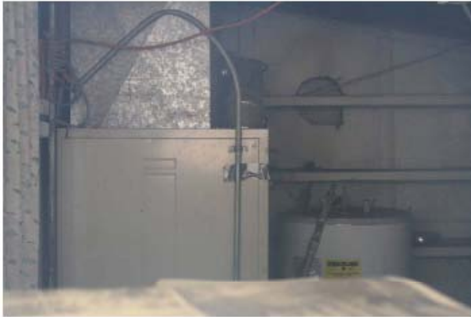
1.Mechanical room-furnace and water heater
