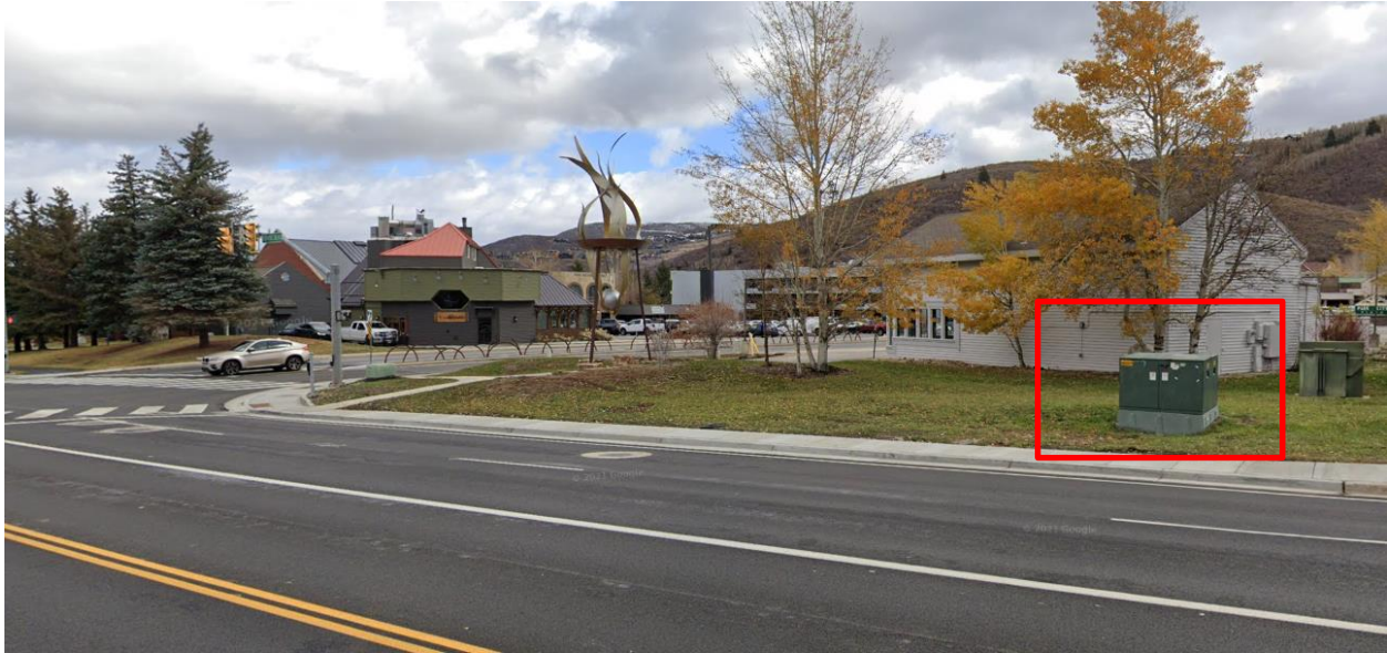
Google Street View of the existing Vault and Switch Gear
